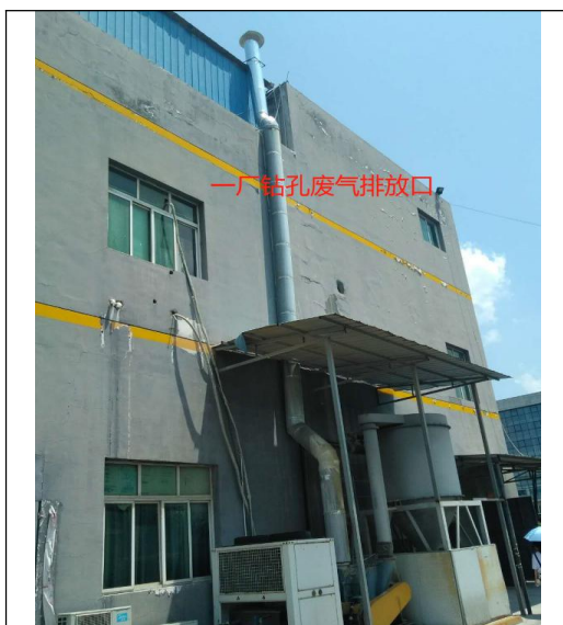
钻孔工序+15m 排气筒
